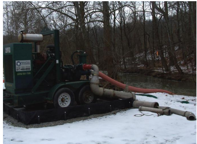
IMAGE 3 RANGE RESOURCES' PUMP SITE CR4 (CHARTIERS CREEK). THE AVERAGE DAILY WITHDRAWAL FOR THIS SITE WAS POSTED AS .2 MILL GAL/DAY. [19]
