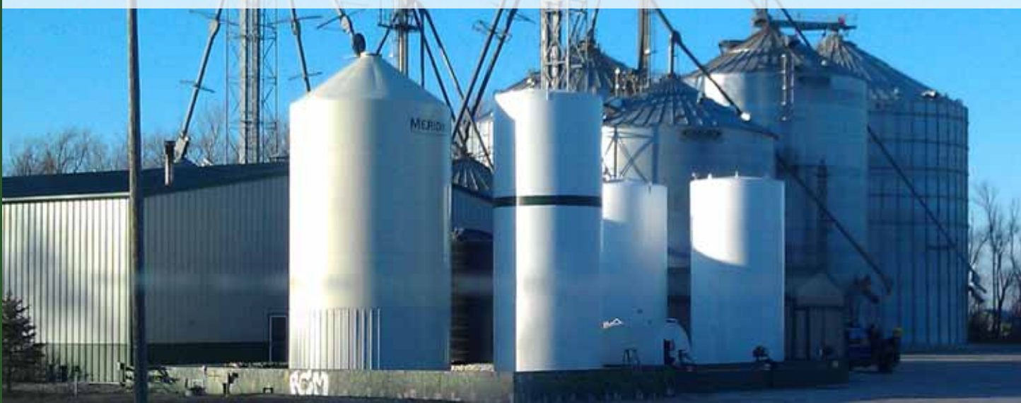
Fuel tanks, located in Richland County, North Dakota, after SPCC Program Outreach. Courtesy of Roxanne Johnson, Water Quality Associate, North Dakota State University Extension
